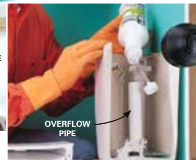
C REMOVE lime deposits
